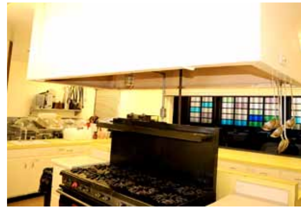
Kitchen Hood Suppression System
